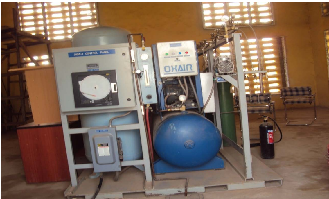
Picture 16: Oxygen Plant at Federal Medical Centre Birnin-Kebbi
