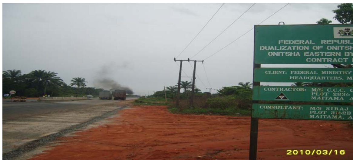
Picture 28: Ongoing Dualization of Onitsha-Owerri Road and Eastern Bypass in Anambra State, Section I
