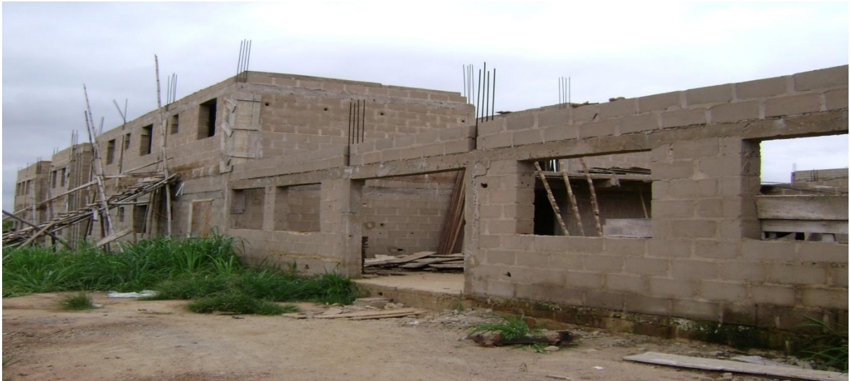
Picture 7: Ongoing Construction of Multi-Ward Complex at Federal Medical Centre Abakaliki, Ebonyi State
