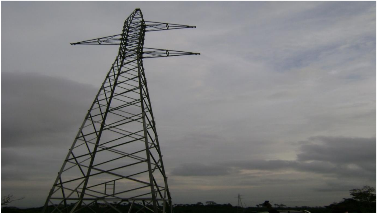
Picture 9: One of the Newly Erected Towers at Umuahia – Mbalano Transmission Line
