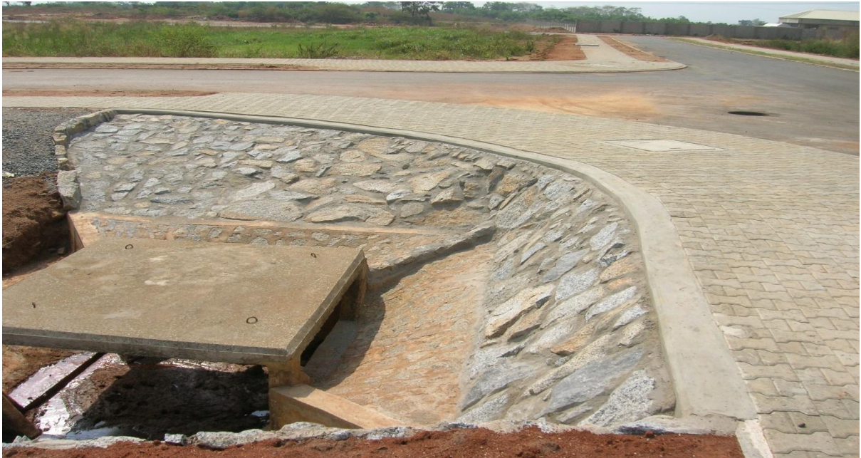
Picture 3: Landscaping/Culvert Works at the Provision of Infrastructure to Katampe District Extension
