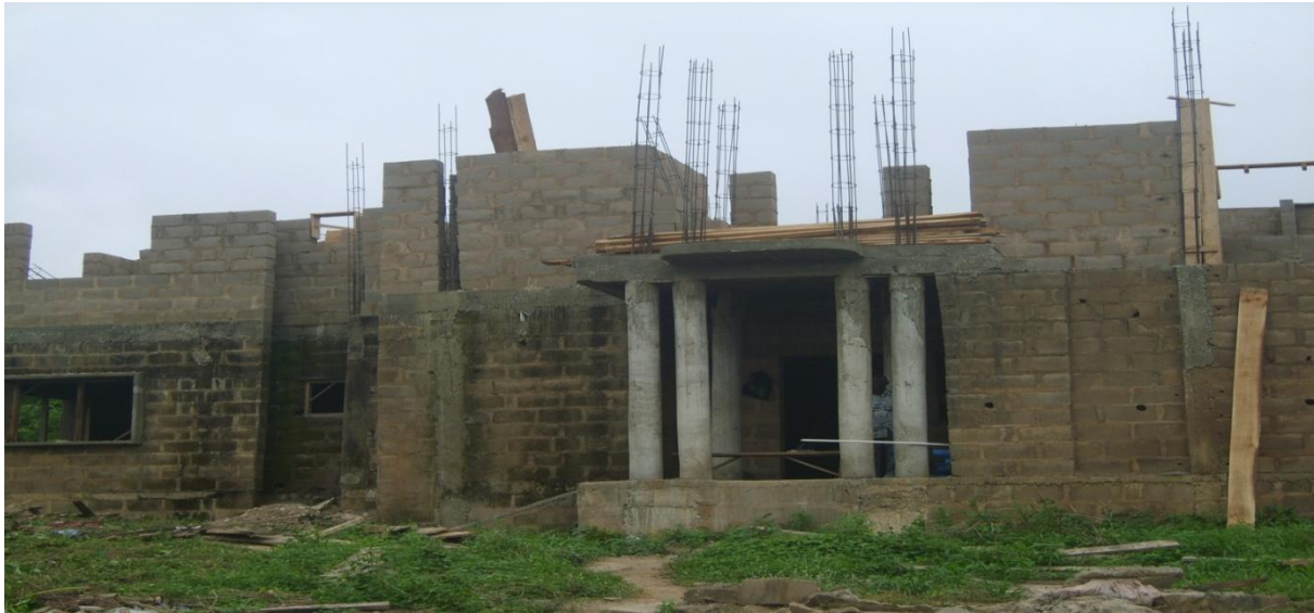
Picture 4: Ongoing Construction of House Officers Block at Federal Medical Centre Abeokuta
