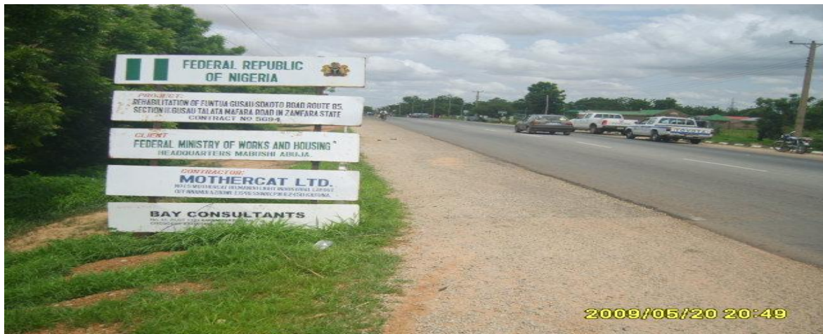
Picture 11: On-going Rehabilitation of Section II of the Gusau–Talata Mafara Road, Zamfara State at 87.73% completion Stage
