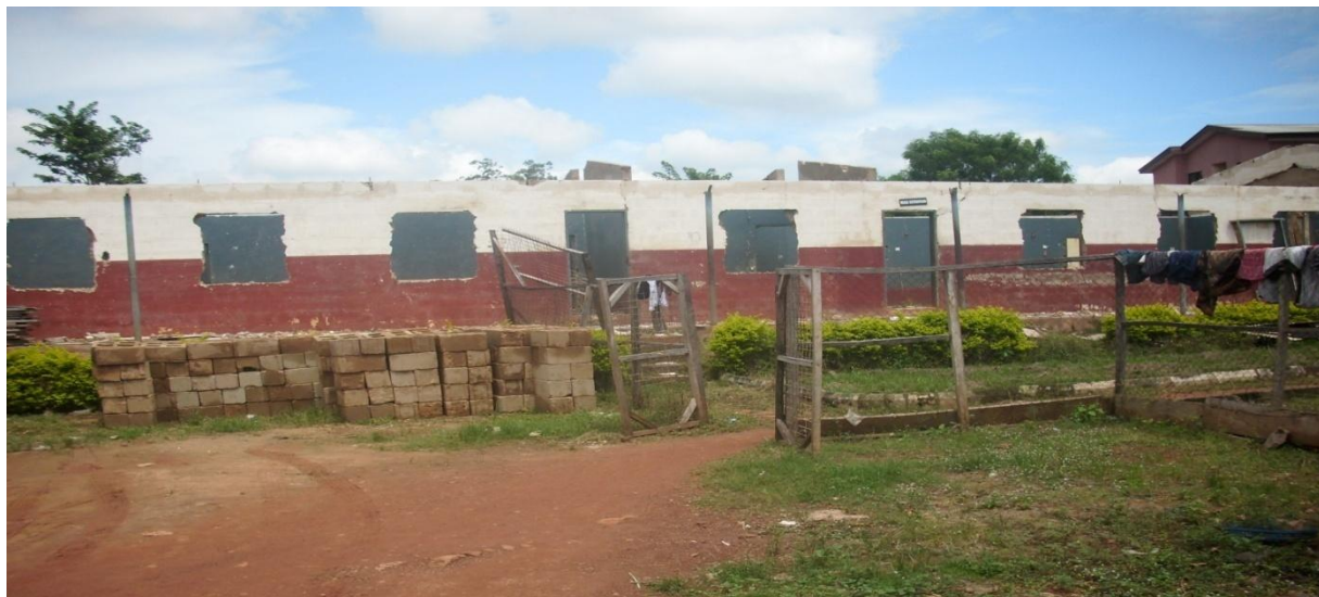
Picture 6: Ongoing Renovation & Upgrading of an Existing Bungalow to a Storey Building, Federal Psychiatric Hospital, Enugu.
