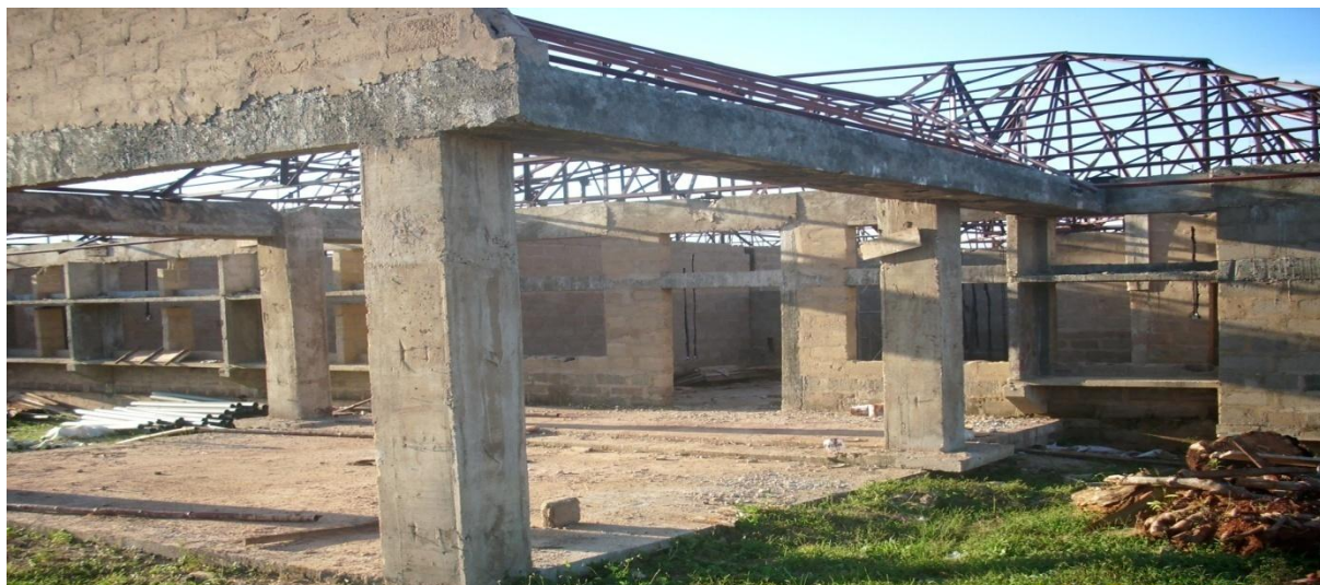
Picture 7: Ongoing Construction of 20-Bedded Spinal Cord Injury Block, National Orthopaedic Hospital, Enugu.
