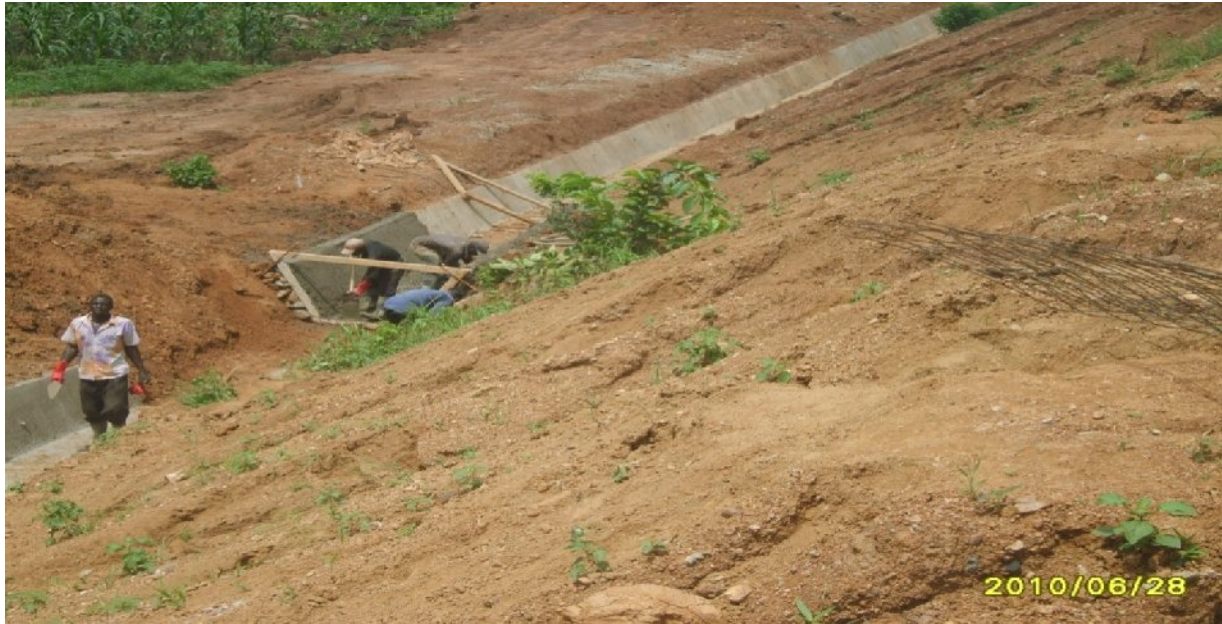
Picture 13: On-Going construction of drainage at dualization of Abuja – Abaji – Lokoja Road, Section II: Sheda Village Junction – Abaji Road
