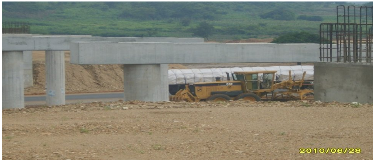
Picture 12: On-going construction of Giri interchange at the dualization of Abuja – Abaji – Lokoja road, Section I
