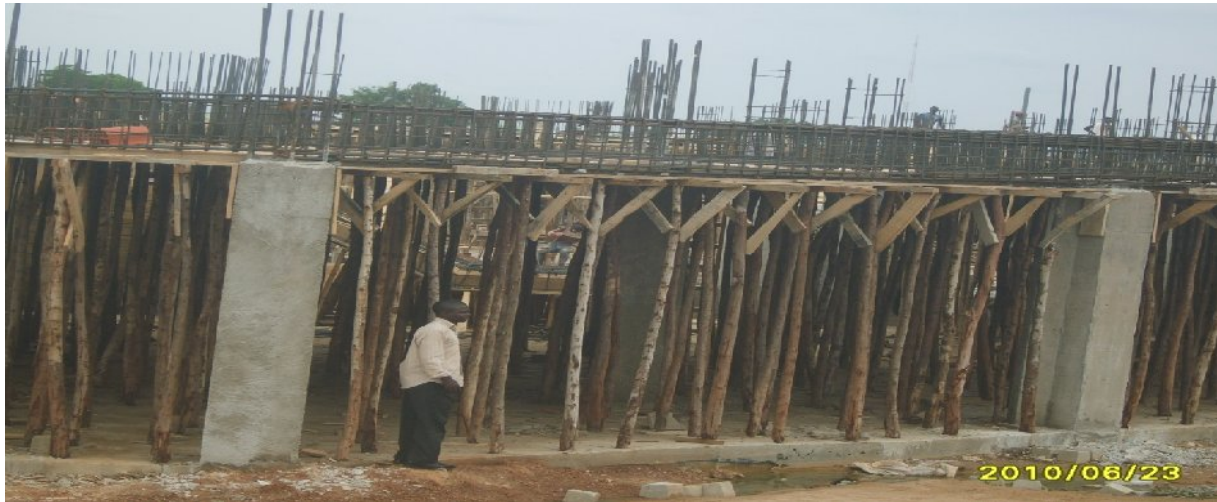
Picture 7: On-going construction of Administrative Building for Lot 1a at the Federal University of Technology, Minna.
