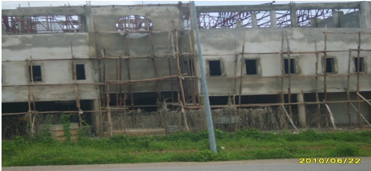
Picture 8: On-going construction of the Central Library at the University of Abuja
