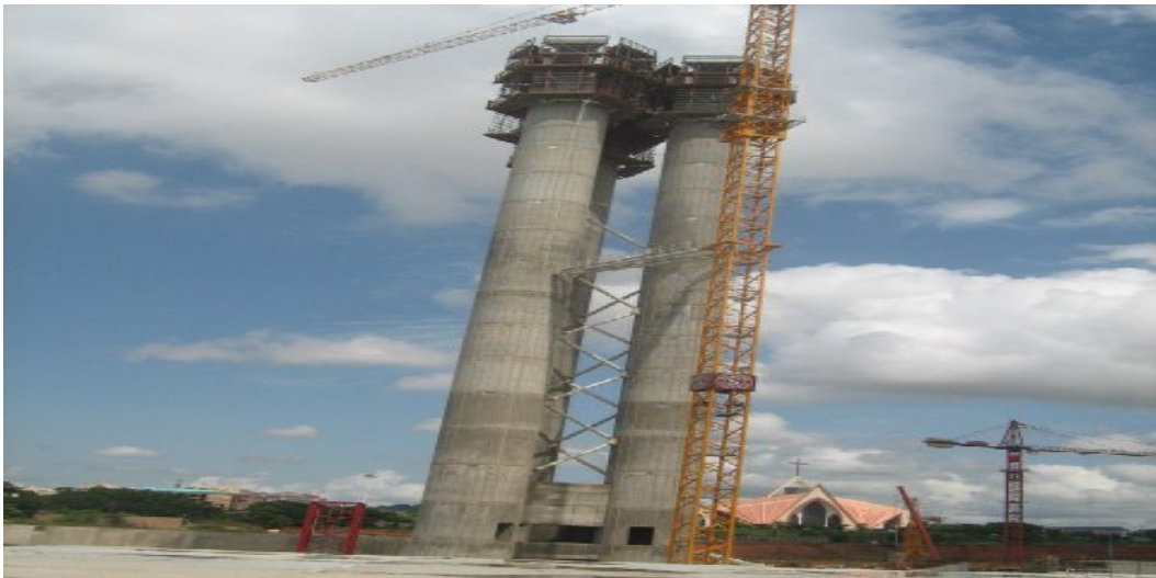
Picture 24(a) & (b): Ongoing work on the Nigeria Cultural center & Millenium Tower
