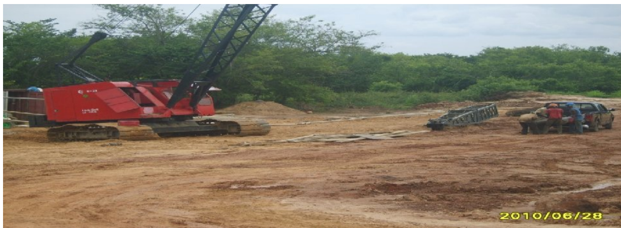
Picture 14: On-going construction work at the dualization of Abuja – Abaji – Lokoja highway, Section IV: Koton-Karfe – Lokoja road
