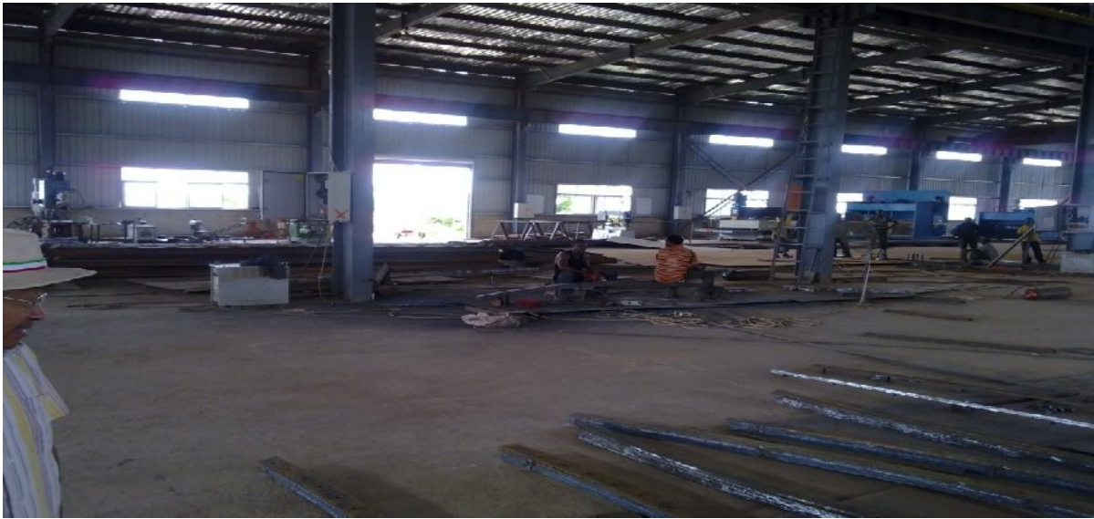
Picture 23: On-going construction site at the Abuja Rail Mass Transit Project, Phase I
