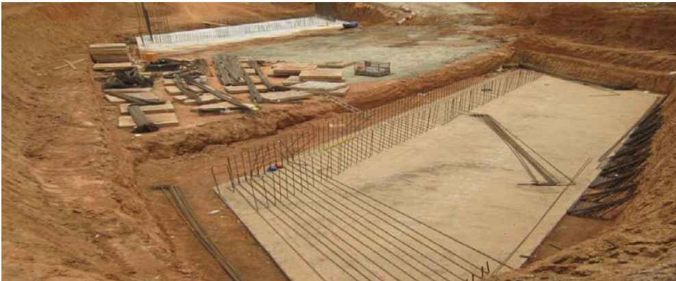
Picture 2: Construction of Underpass Bridge in progress around the City Gate Arena
