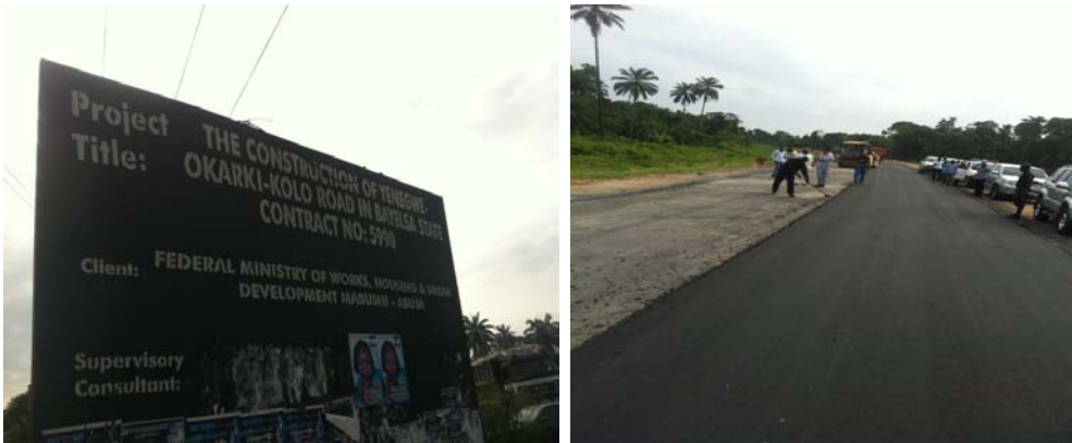
Picture 8: Asphalt work in progress at Yenegwe – Okarki – Kolo Road, Bayelsa State.
