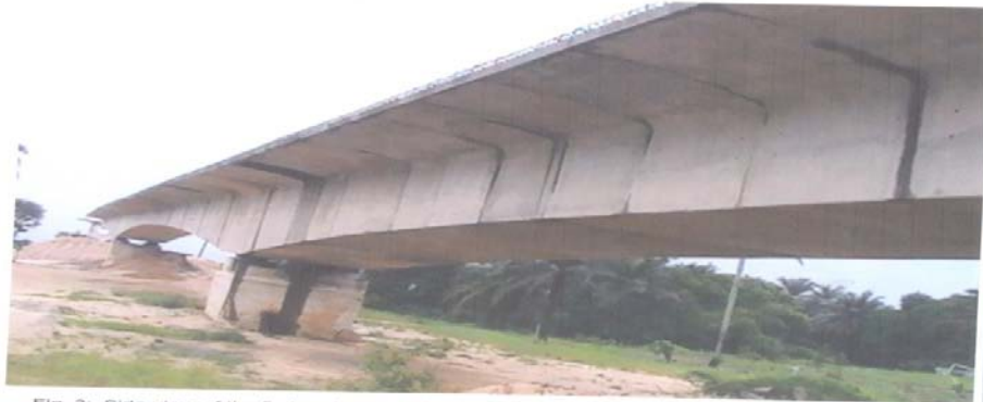
Fig. 3: Side view of the first and second Span of the Bridge from Bodo side
