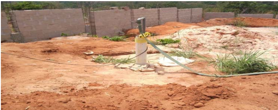
Picture 16b: Perimeter fencing and borehole works at the Ojoto sub -station under construction
