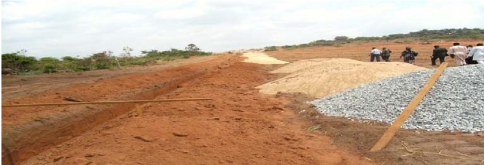
Picture 16a: On-going work at the construction of 2 x 132KV Line Bay at Ojoto
