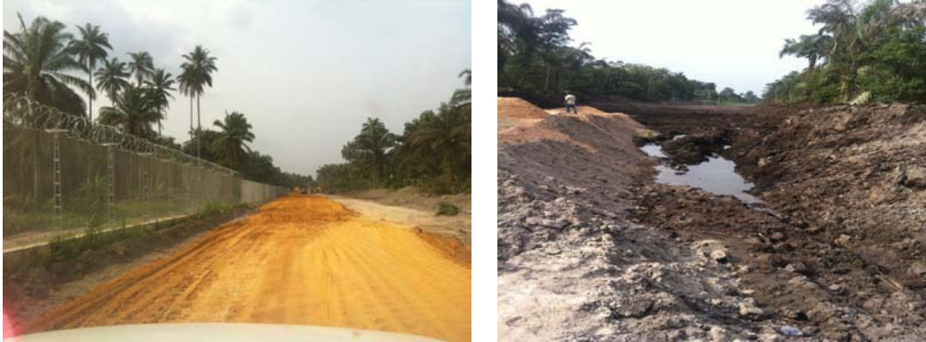
Picture 18(a): On-going construction of Bi-Metal Fence & Asphalt Road at P/Harcourt Airport (b) Swampy Portion of the road that requires heavy sand filling
