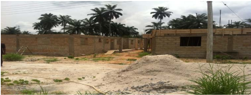
Picture 34: Suspended Construction of 1no. 8 – Man Rank and File Quarters (Storey type)
