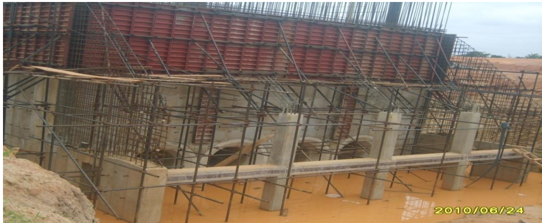
Picture 5: On-going Construction Work at Intake Tower (Kontagora Auna Dam and Irrigation Project)
