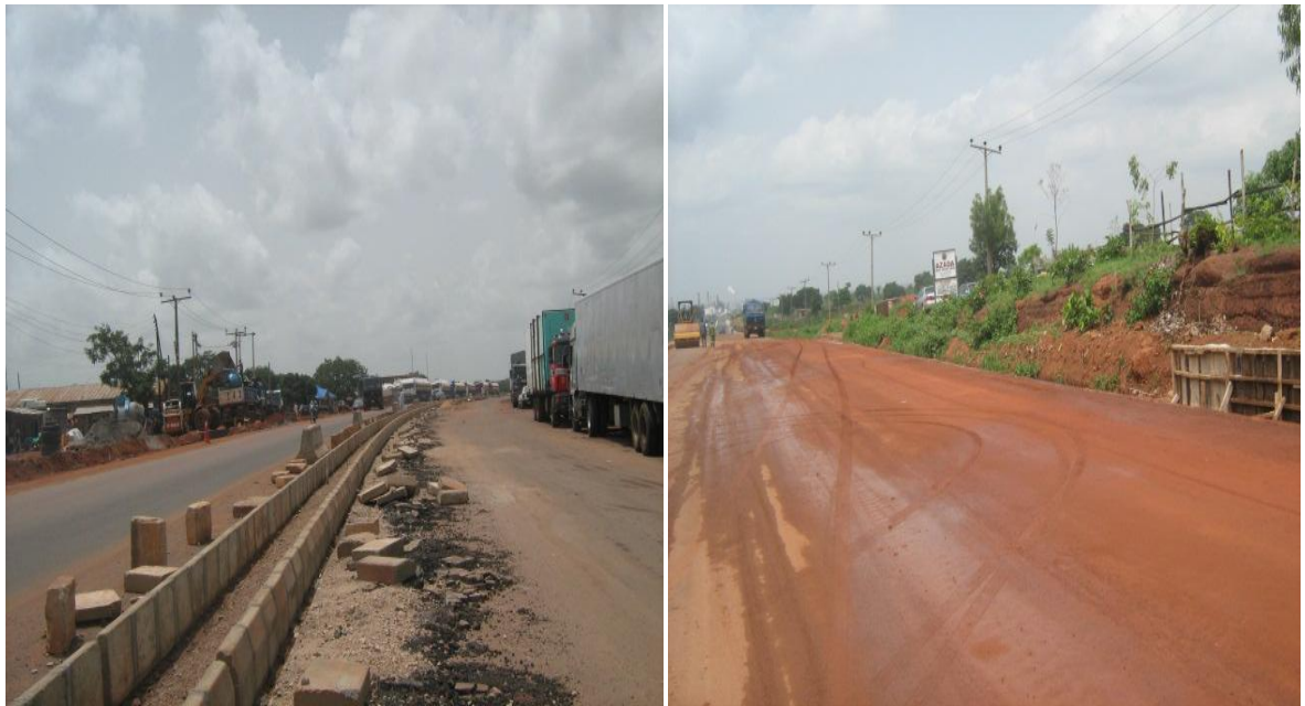
Picture 2: a. Rehabilitation of Refinery – Kachia Road b. Rehabilitation of Access Road to Kaduna Refinery
