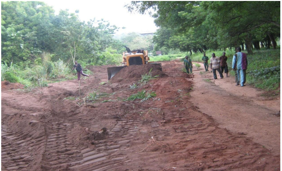
Picture 18: Ongoing Construction of 0.45km Asphalt Road at the Neuro- Psychiatric Hospital, Abeokuta.
