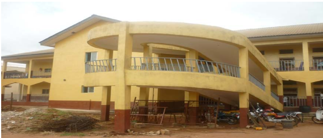
Picture 14: Ongoing Renovation work at the Temporary site at Nnamdi Azikiwe Teaching Hospital, Nnewi
