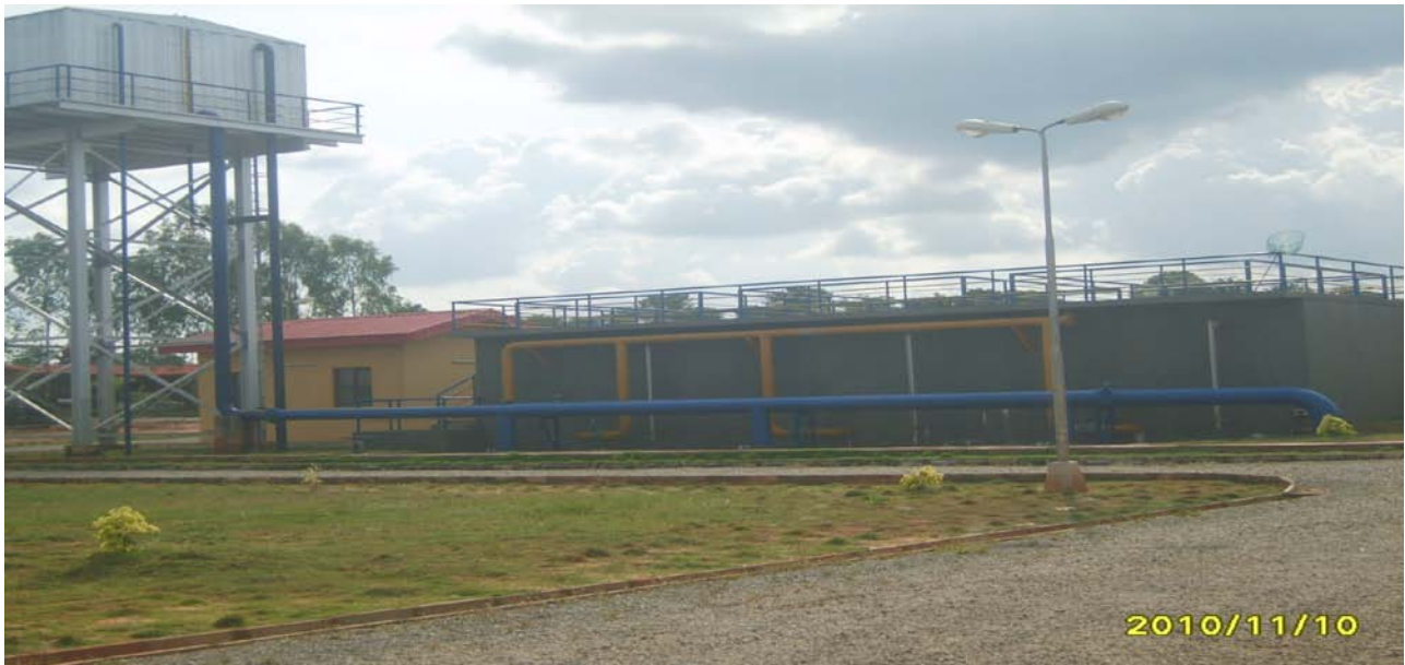
Picture 30: Construction of Overhead Tank and Water Treatment Plant at Northern Ishan Regional Water Supply
