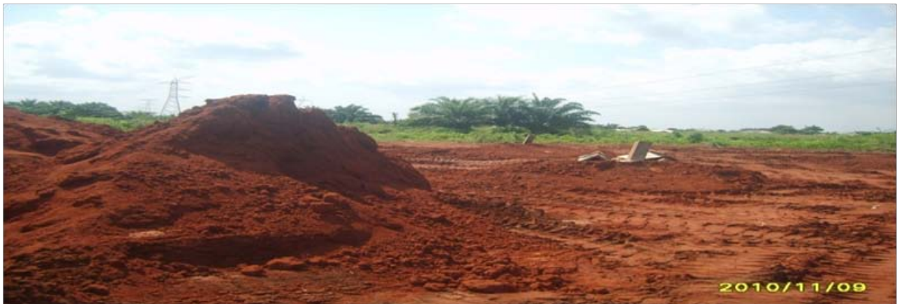
Picture 19: The 2 nd and 3 rd Benin – Onitsha Transmission Lines meeting point
