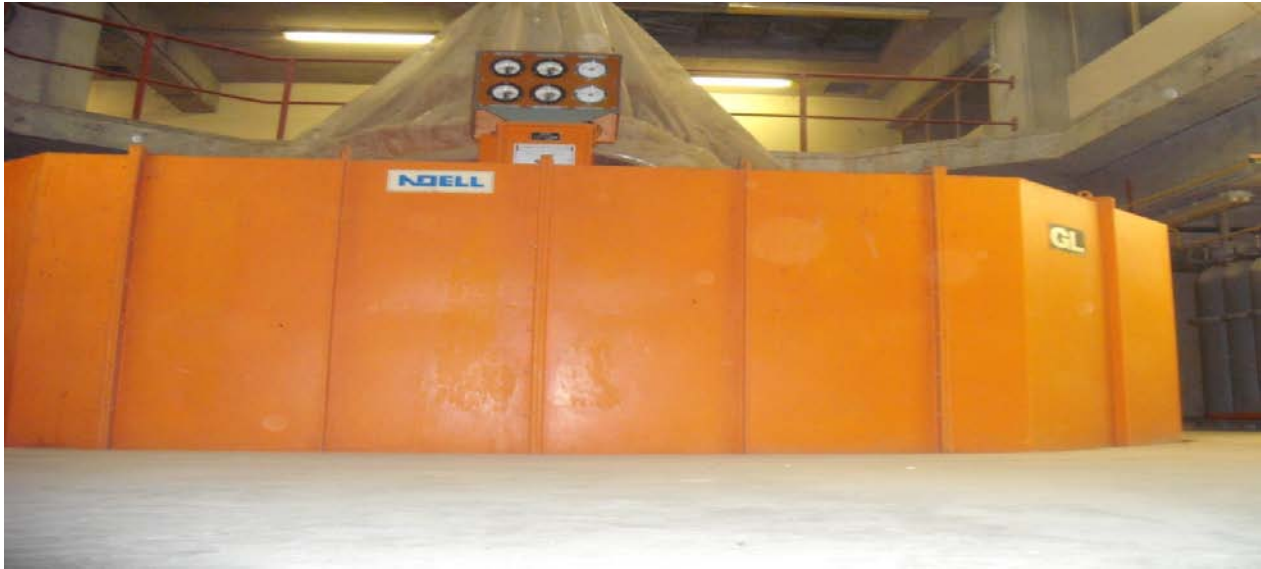
Picture 17: One of the 3 Turbines at Oyan River Hydro Power Station
