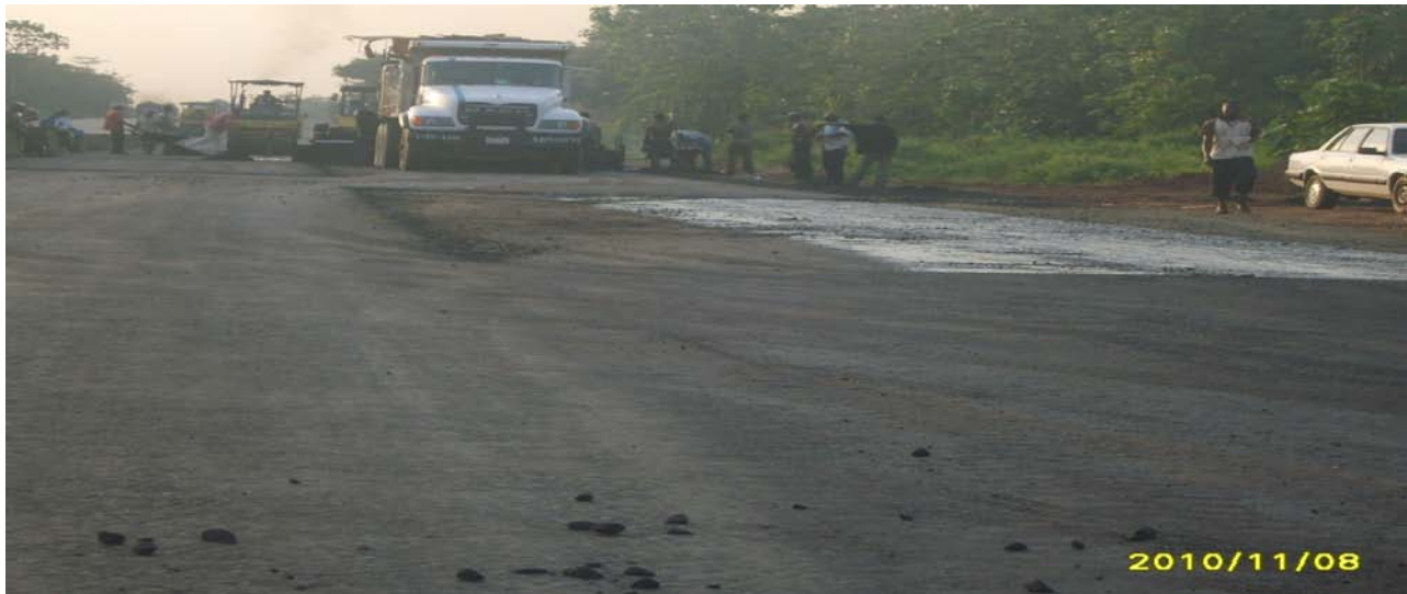
Picture 26: Rehabilitation Work at a Section of Benin-Shagamu Dual Carriageway, Benin-Ofosu Section (Edo/Ondo State Boarder) Edo State, C/No. 5900
