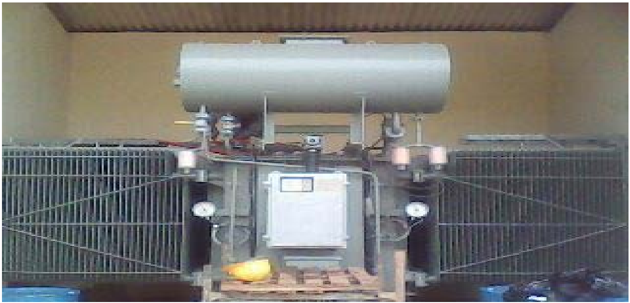
Picture 5: One of the 3x15 MVA Transformers at Guzape District
