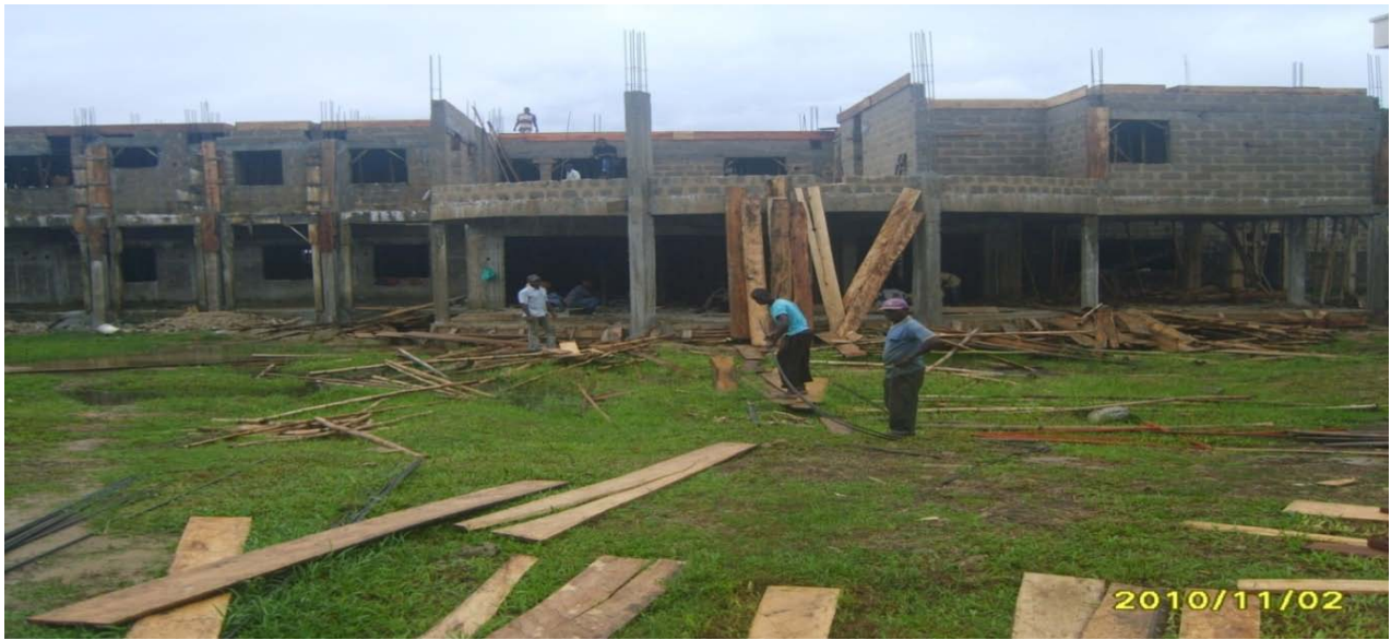
Picture 15: Front View of the Construction of the One-Storey Obstetrics and Gynecology Block at the Federal Medical Centre, Yenagoa.
