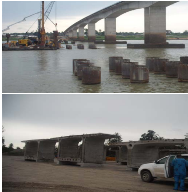
Picture 1: East West road (Section 1) - Casting of Piles at the Forcados River
