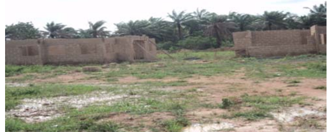
Picture 8: Construction of Engineer's quarter which was stalled at the Ivo Dam project
