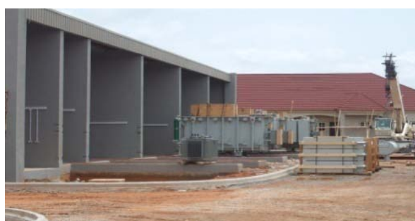
Picture 17: Ongoing sub-station (building) and installation of transformer at the Karmo district.
