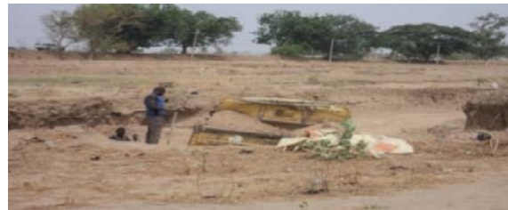
Picture 11: A Portion of uncompleted dyke work evacuated by neighbouring communities at the abandoned Chouchi Irrigation project
