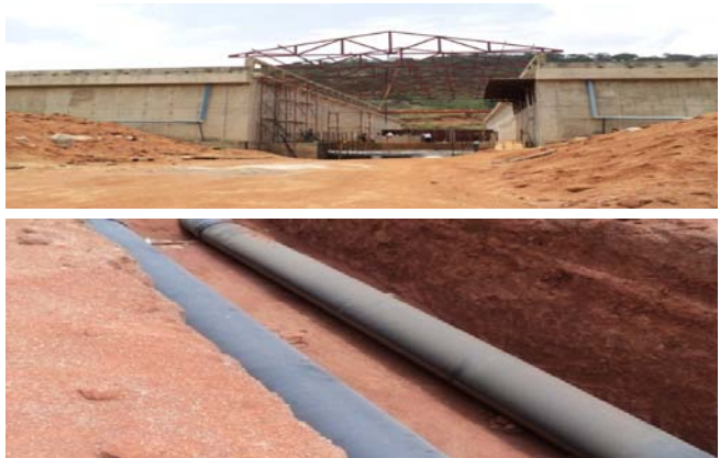
Picture 15: Tank 1 almost completed & laying of 10km pipelines at the project site.
