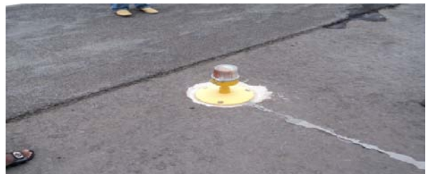
Picture 6: Completed Runway Extension & one of the Airfield lighting at Enugu Airport
