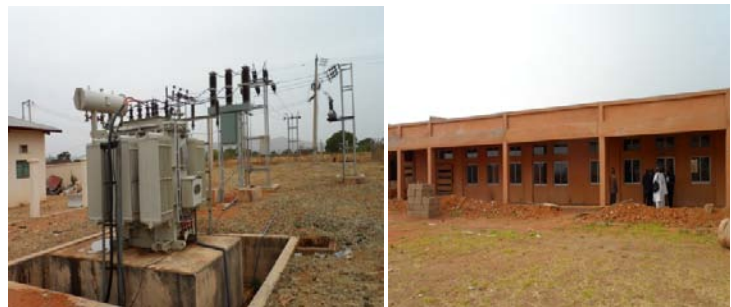
Picture 34: Completed Laboratory and Newly installed Electricity Transformer
