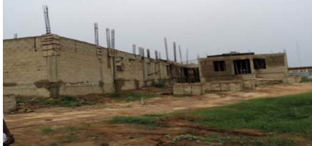
Picture 35: Construction of CT Scan Building at University of Uyo Teaching Hospital.
