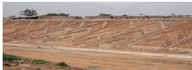
Picture 14: Laying of tracks & Part of Erosion protection works which was stalled at the site.
