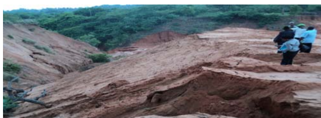
Picture 3: Part of the eroded spots requiring & reduction of existing slope/earthworks in progress at Isikwato Erosion site
