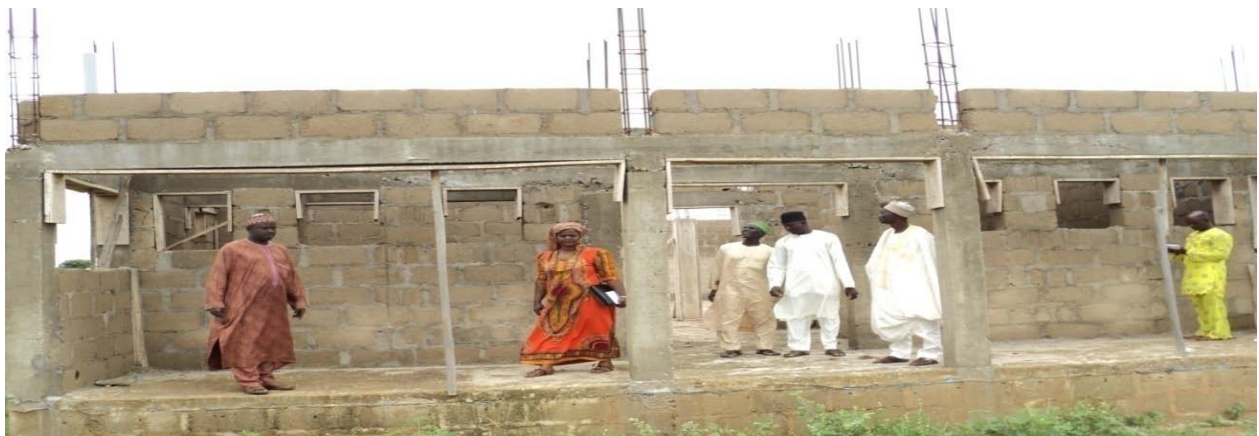
Picture 4.31(b): Construction of Male hostel which was stalled at the Project site
