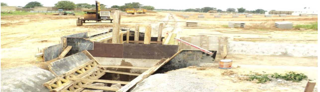
Picture 4.5(b): Drainage works around the Flyover Bridge of the Kano Bye-pass
