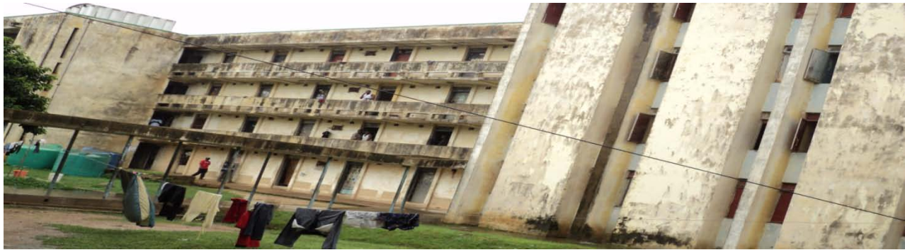
Picture 4.36: The dilapidated students' hostel at Kongo campus requiring urgent rehabilitation ABU, Zaria
