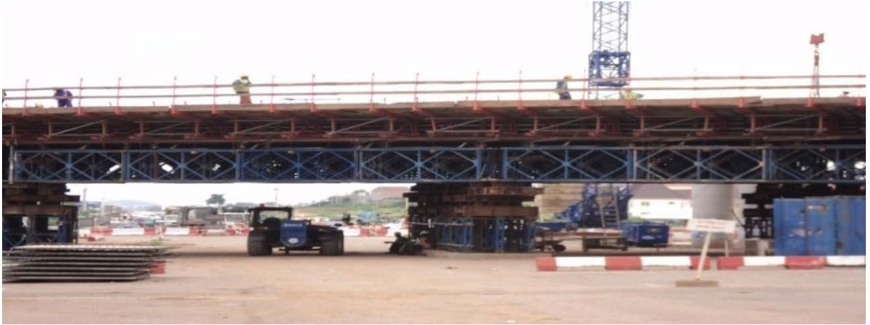
Picture 4.1(a): Work in progress at Ring Road 2/N5 interchange (Jabi/Gwarinpa Area)
