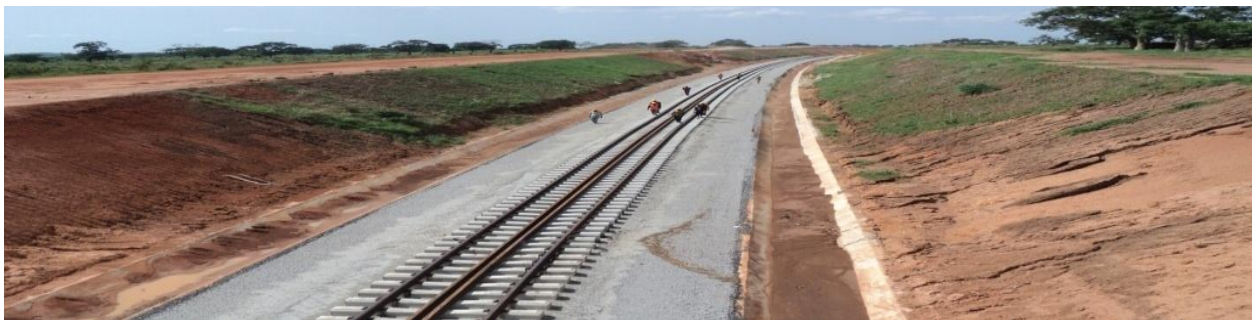
Picture 27: Completed portion of the Abuja (Idu) Kachia Rail Line around Kuchubun-Asham village
