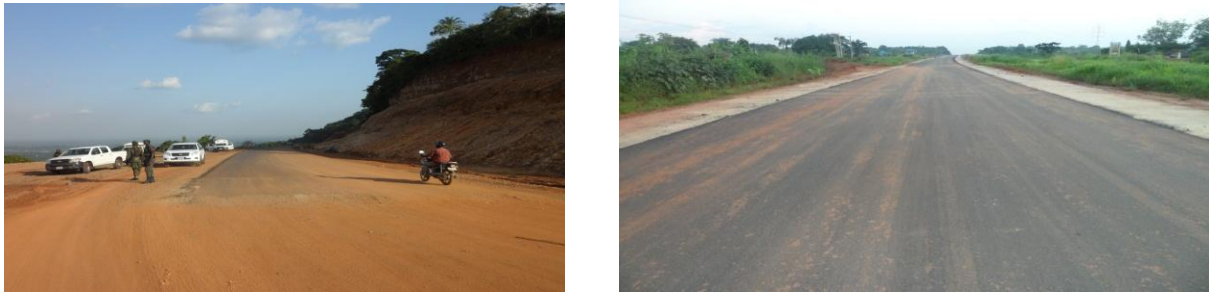
Picture 6: On-going works and completed portion of the road at Orji-Achi-Mmakwu-Augu-Ndiabo Mpu-Akazeze.
