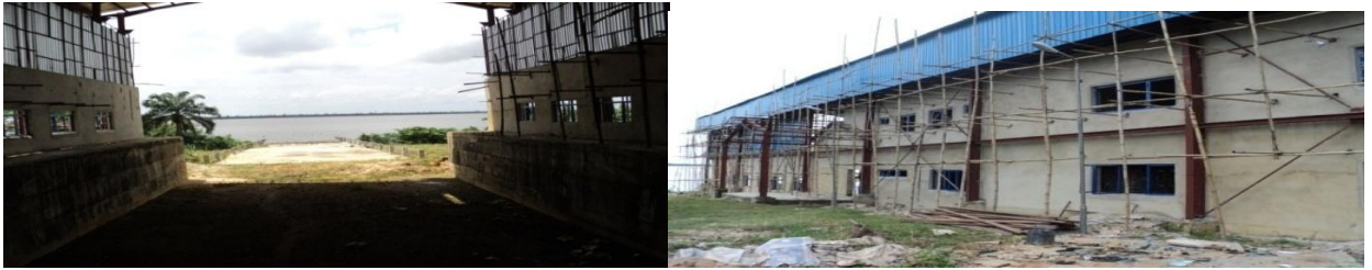
Picture 25: Completed Spillway and on-going construction of the boat/ship maintenance workshop at Oron
