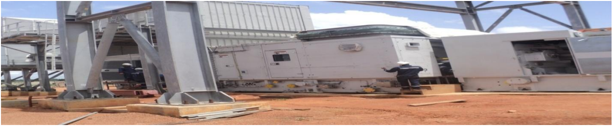
Picture 21: Ongoing realignment of Gas Turbine at 215 MV Dual Fired LPFO/Gas Power Plant, Kaduna
