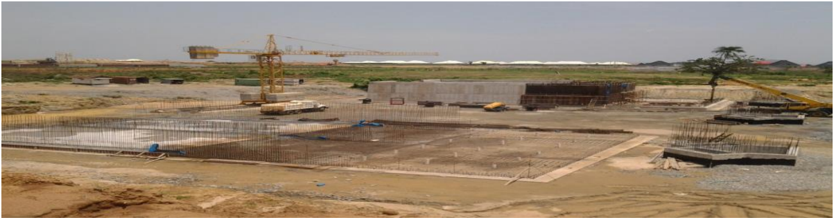
Picture 3: On-going construction work of concrete line drain at the Abuja Technology Village.
