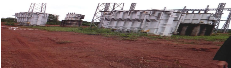
Picture 32: 2No. 2x30/40 MVA and 2no auxiliary transformer installed.
