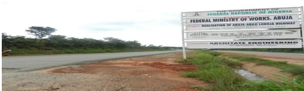
Picture 2: Newly Constructed Portion at Km 0 of the Dualization of Abuja - Lokoja Road Section III (Abaji – Kotonkarfi)
