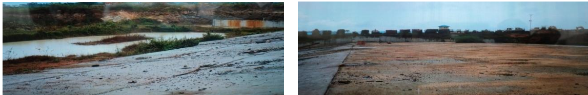
Picture 27: The On-going construction of Spillway Excavation and foundation grouting at Ogbese Multi-Purpose Dam
