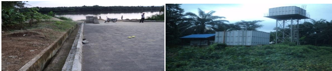
Picture 30: Erosion control works at Ikom. Pic 2: Completion of overhead tank work at Nselle and Njematop
