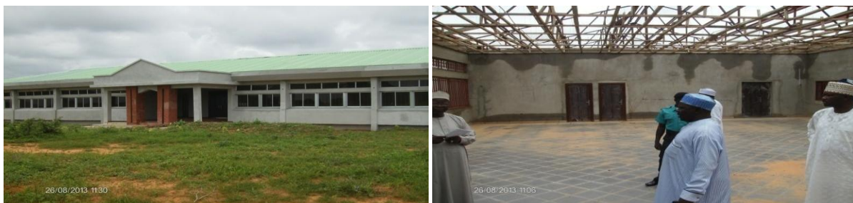
Picture 23: On-going Construction of the Department of Architectural Technology building & the area affected by storm being re-roofed.
