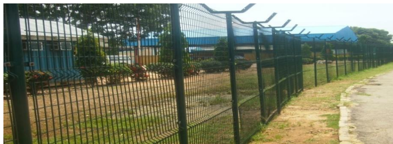
Picture 15: Part of the completed bi-metallic fence installation around the Nigerian Airspace Management Agency Division of the College.
