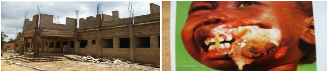
Picture 16a: On-going Construction of Administrative & Visiting Surgeons' Villa; Picture 16b: One of the cases treated at NOMA Children Hospital, Sokoto
