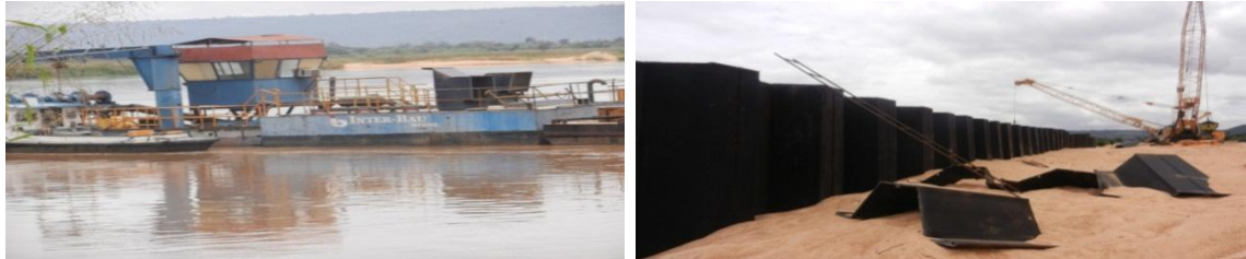
Picture 12: One of the Dredging boats, a completed key wall and vibrator at River Port Lokoja
