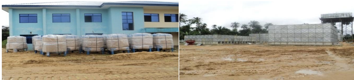
Picture 31: Completed Admin block and 13nos.of water filtration. Pic2: 5nos.of steel elevated water tanks
