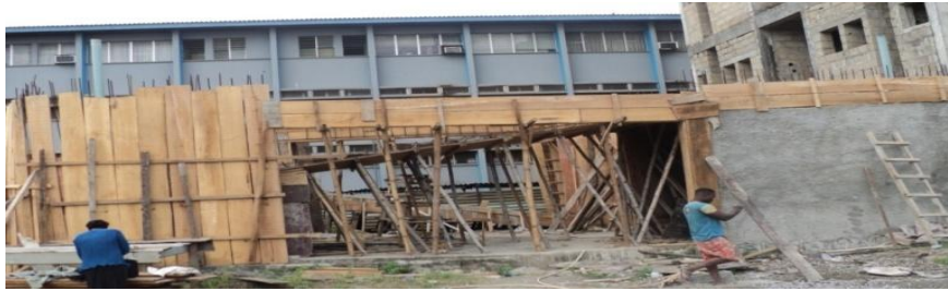
Picture 18: On – going Construction of Construction of Interns Staff Quarters at Lagos University Teaching
