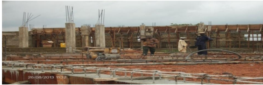
Picture 24: Setting of beams and DPC works for Department of Building Technology in progress at the Polytechnic site.
