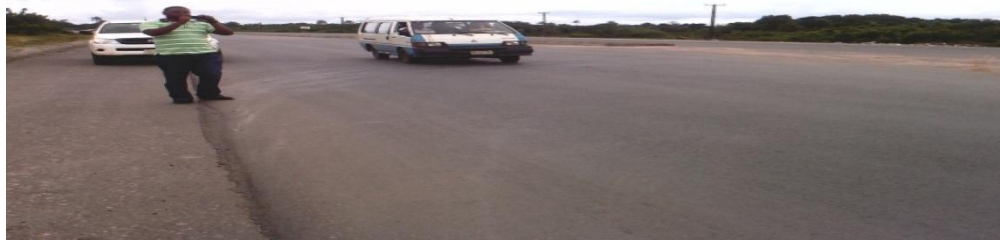
Picture 35: A portion of road completed at Owerri- Elele in Imo State
