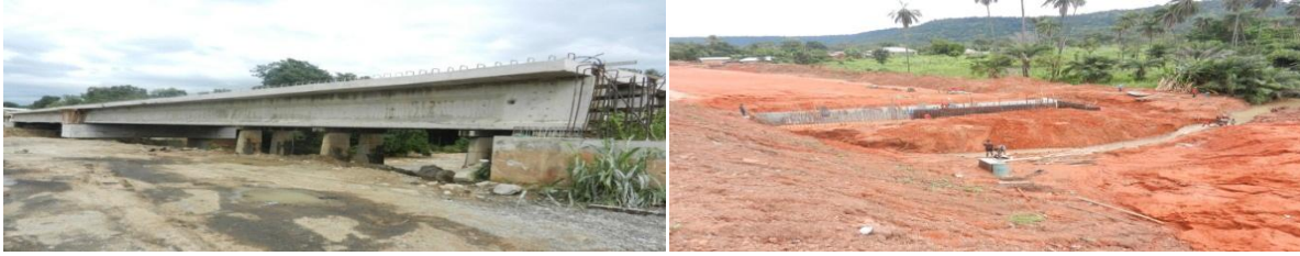
Picture 3: On-going Construction of Bridge at Section IV of Abuja- Lokoja (Kotonkarfi–Lokoja)
