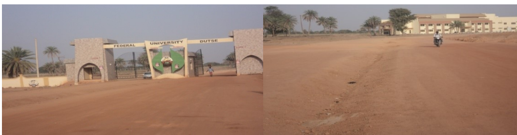
Picture 39: On-going Construction of Access Road from the Main Gate to the Senate Building
