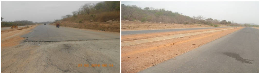
Picture 11: Part of the Sectional Failures & Wearing Course of the Obajana-Okene Road Project
