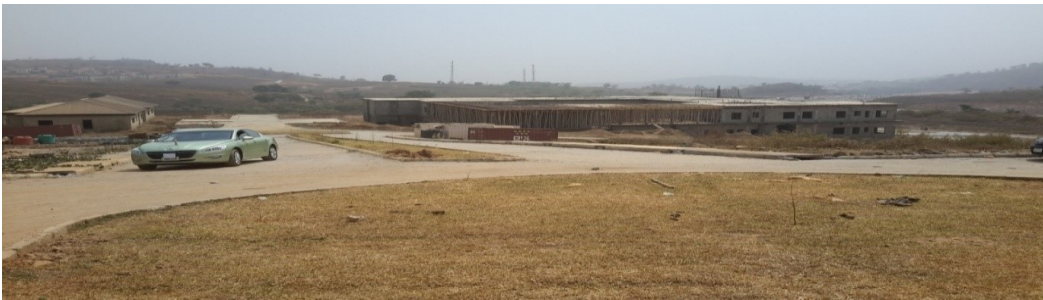
Picture 6: Construction of Armed Forces Hospital and Research Centre Mogadishu Cantonment, Abuja
