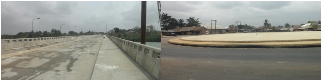
Picture 10: Ongoing Bridge Construction and Completed Round About at Section IV (Eket-Oron)
