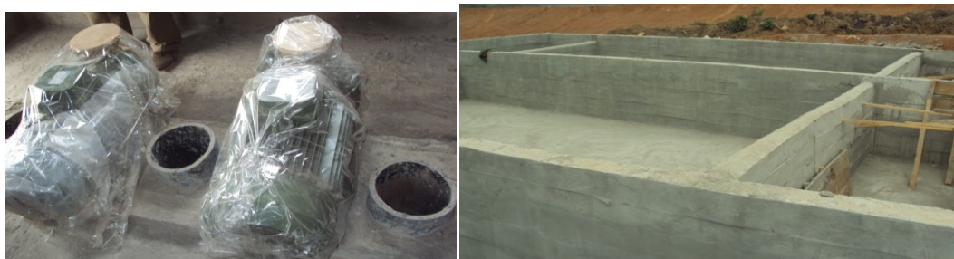
Picture 27: Ongoing Construction of Water Treatment Plant at Oko Town, Surulere LGA Ogun State
