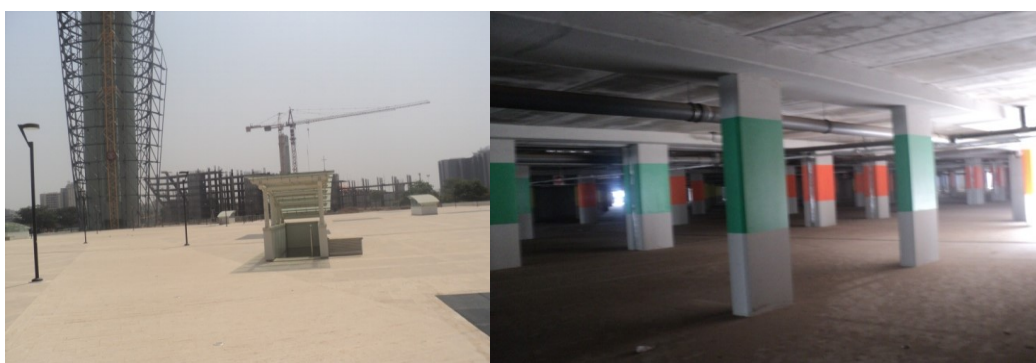
Picture 21: Ongoing Construction of Millennium Tower & Underground Car Parking Space at the Cultural Centre
