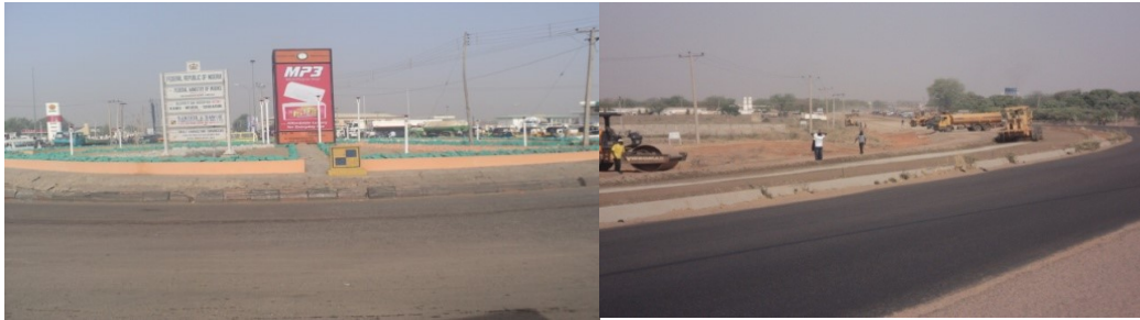
Picture 14: On-going Construction of Kano – Wudil – Shuarin Section of Kano-Maiduguri Road, Section I
