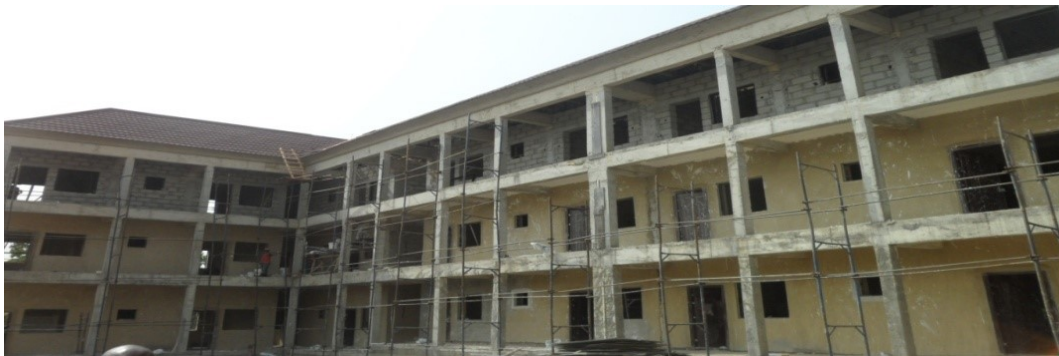
Picture 5: Ongoing Construction of 2 Storeys Building for Students Hostel at Defence Intelligence Agency (DIA), Karu
