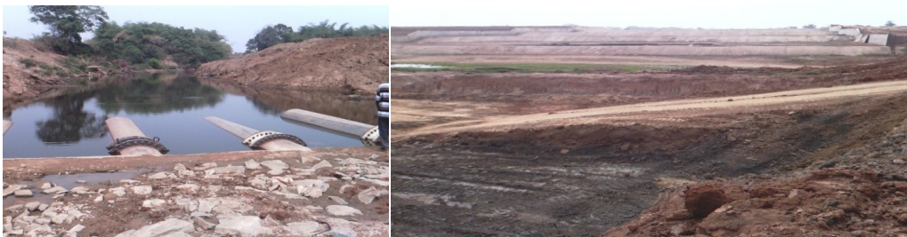
Picture 24: Penstocks Pipe for Hydropower Inlet/Outlet Structure and Broad Crested Concrete Spillway
