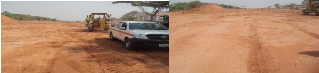
Picture 20: On-going Construction for the Extension of Inner Southern Express (ISEX), Abuja
