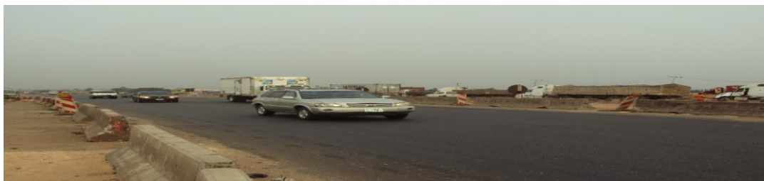
Picture 15: Completed Portion of Binder Work at the Rehabilitation and Expansion of Lagos – Ibadan Expressway, Section 1 (Lagos – Shagamu)
