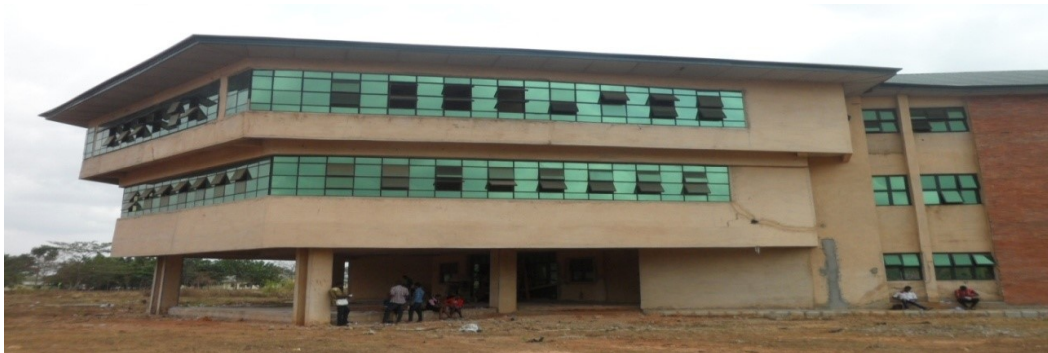
Picture 38: Ongoing Construction of the Faculty of Agriculture at University of Benin
