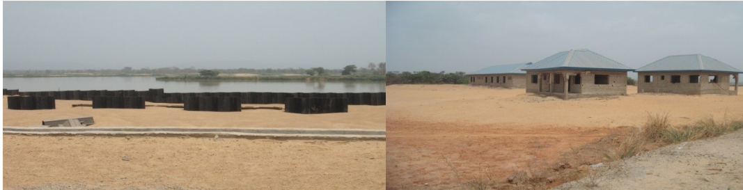
Picture 1: Part of Steel Sheet Pile Quay Wall & Staff Quarters / Police Station at River Port Lokoja
