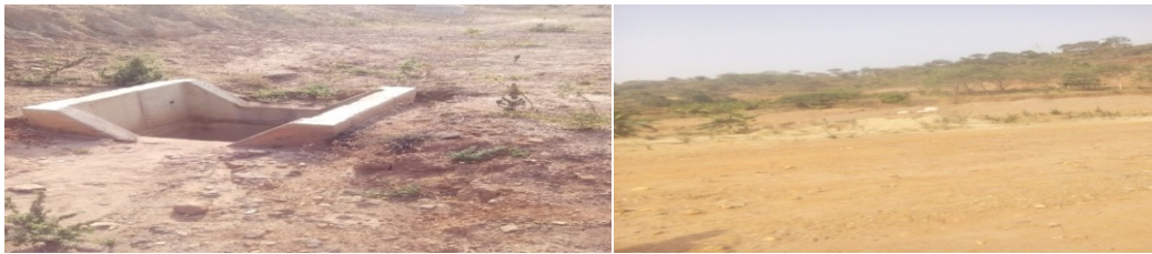
Picture 19: Part of Surface Water Drainage and Earth Works at Sub-Section 105 of the Project
