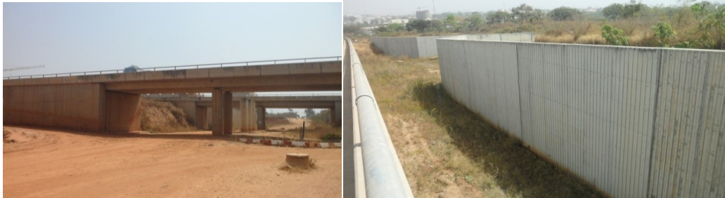
Picture 17: Completed Underpass and Retaining Walls on Roads B6, B12 and Circle Road
