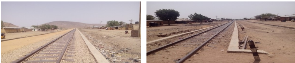
Picture 3 : Ongoing Ballast Retainace and Erosion Control along Gombe-Bajoga Axis of Track Rehabilitation (Kuru- Maiduguri)
