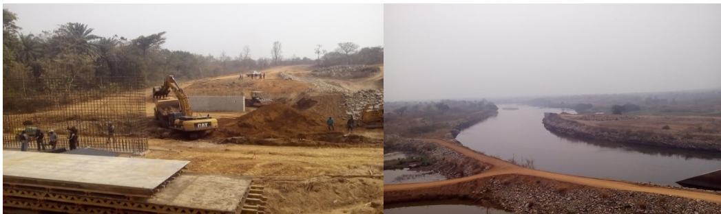
Picture 23: On-going Construction of Access Road and Completed Cofferdam Embankment at the Project Site
