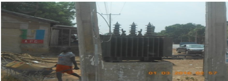
Picture 25: One of the Transformers Installed at Ikumbu Community
