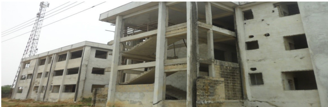
Picture 31: Ongoing Construction of the General Out Patient Department at University of Uyo Teaching Hospital
