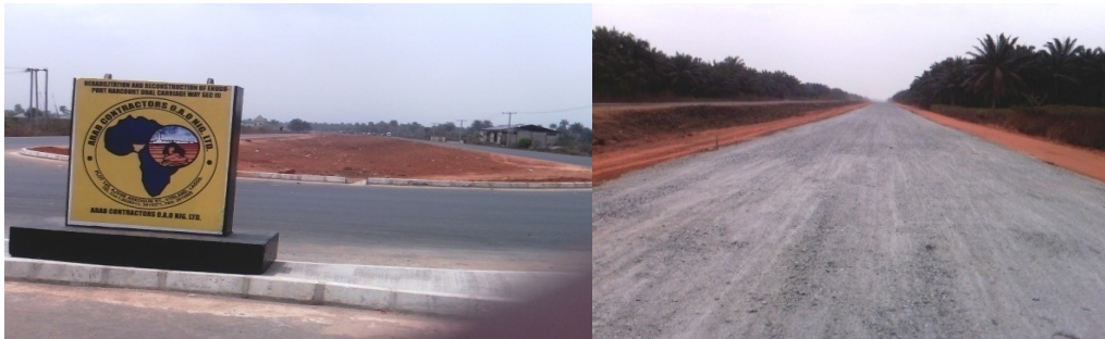
Picture 13: Completed Portion and Ongoing Works at Enugu-Port-Harcourt Dual Carriage Way, Section II
