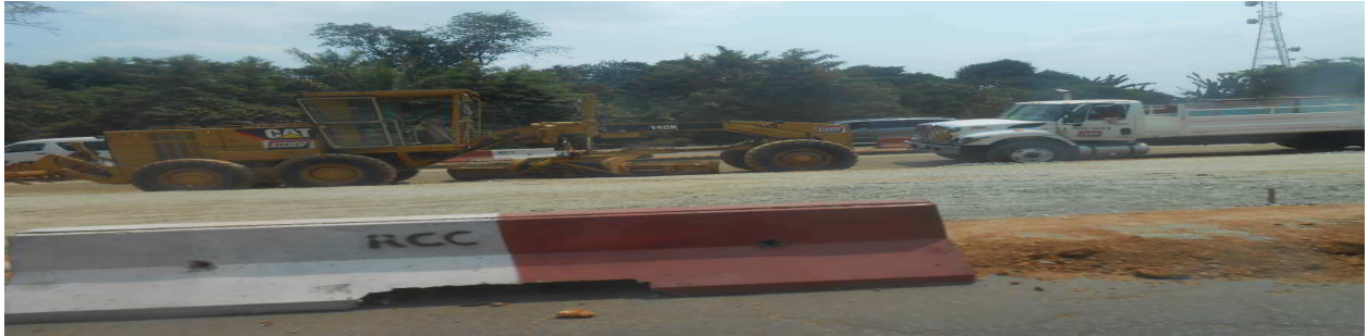
Ongoing Construction Work at the Lagos Ibadan Expressway Source: Project Monitoring by CWP, February 2014
