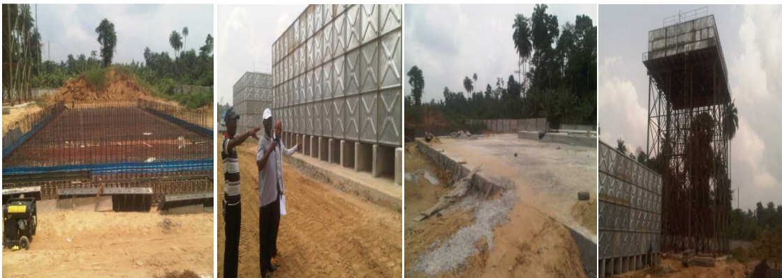
Images of Booster Station at Emeyal and the Safety Tank Source: Project Monitoring by CWP, February 2014
