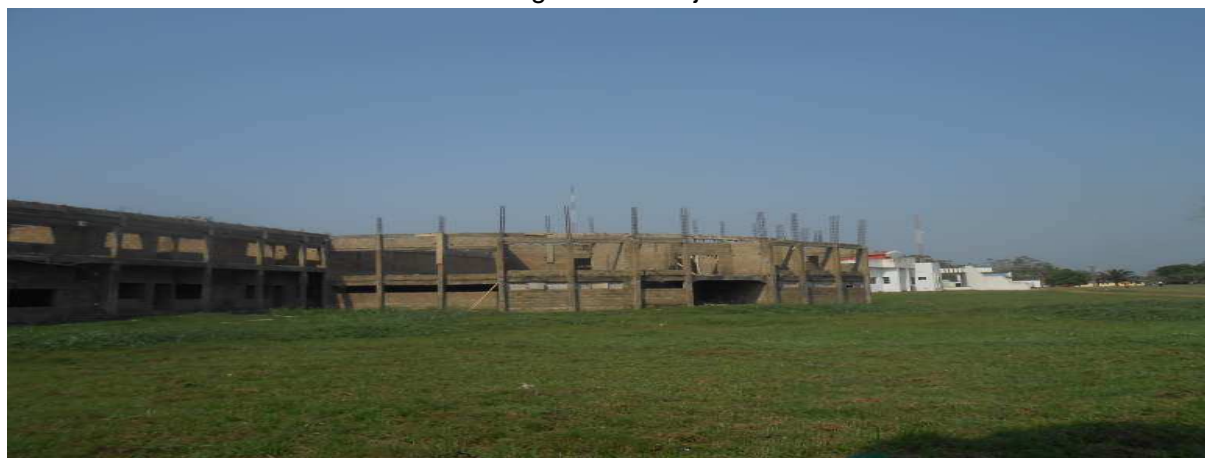
Ongoing Construction Of Academic Board Room Source: Project Monitoring by CWP, February 2014
