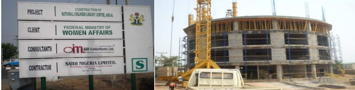
On-going Construction work at site of National Children Library Centre, Abuja Source: Project Monitoring by CWP, February 2013
