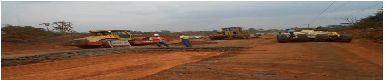
Ongoing construction work at the Akure-Ilesha Road Source: Project Monitoring by CWP, February 2014
