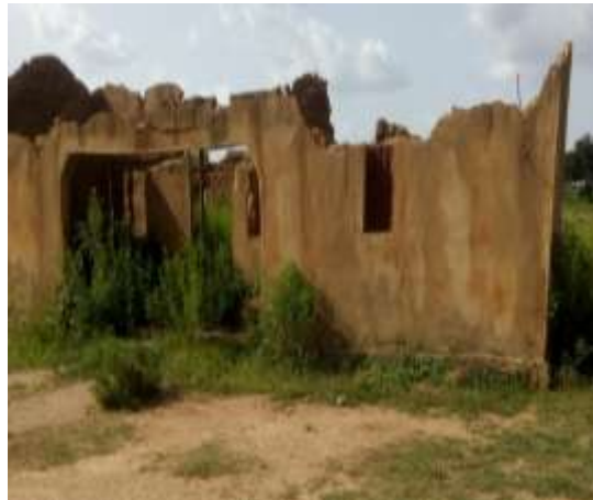
Picture 24: The Old Building that Collapsed
