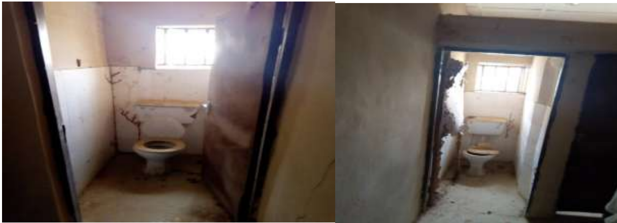
Pictures 52 and 53: Unkept Toilets at Doka Marshi PHCC
