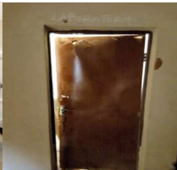
Picture 55: Door Eaten by Termites
