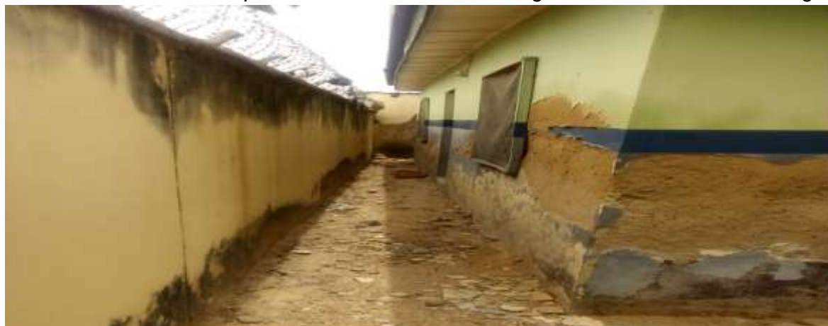
Picture 95: A dilapidated wall of the PHC showing the state of the PHC building
