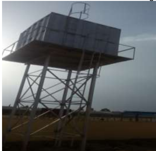
Picture 87: PHC's Borehole-Not working
