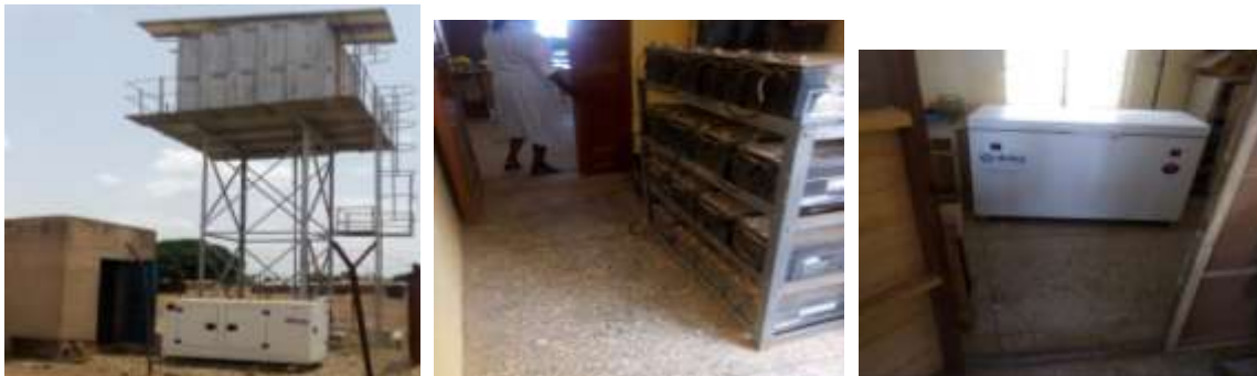
Picture 73: Generator, Overhead Tank, Solar Batteries and Fridge for the Facility
