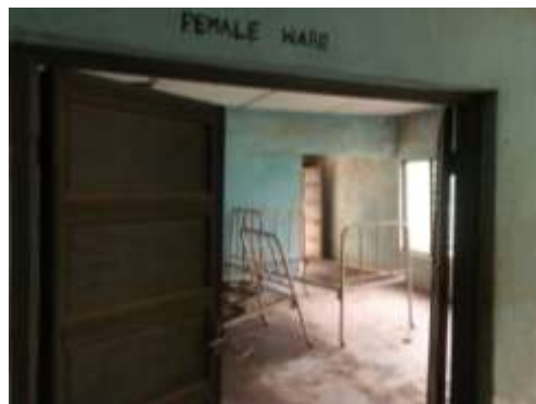
Picture 4: Dilapidated Female Ward
