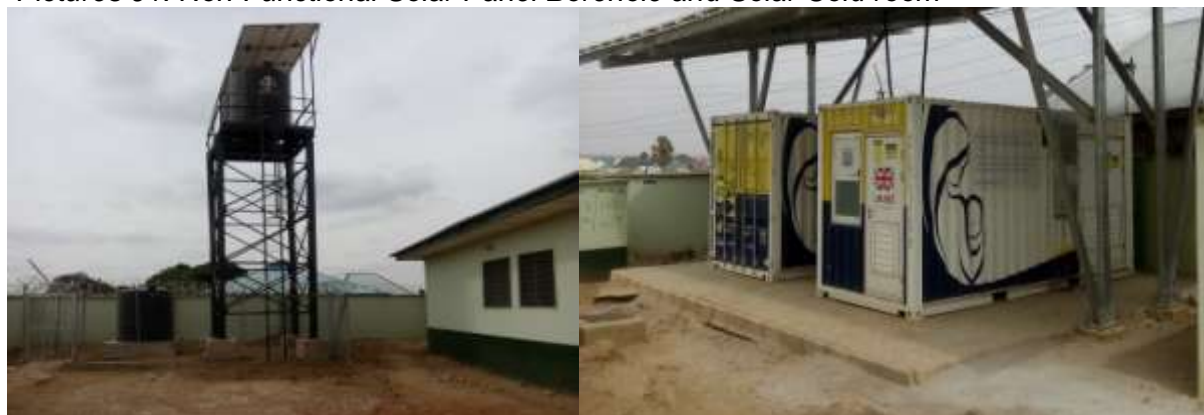
Pictures 91: Non-Functional Solar Panel Borehole and Solar Cold room
