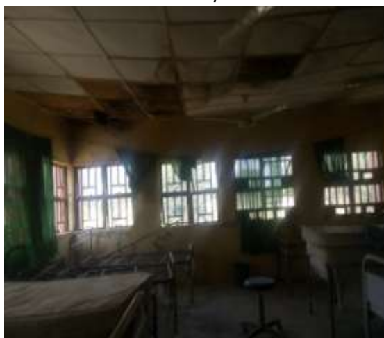
Picture 28: The Dilapidated Wards
