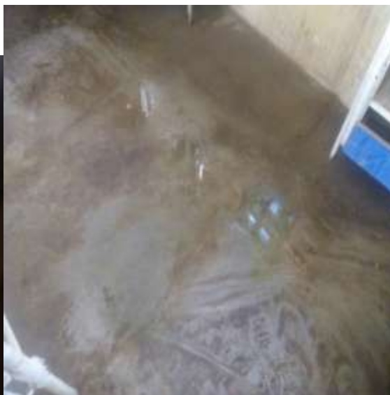
Picture 30: Water-logged Floor
