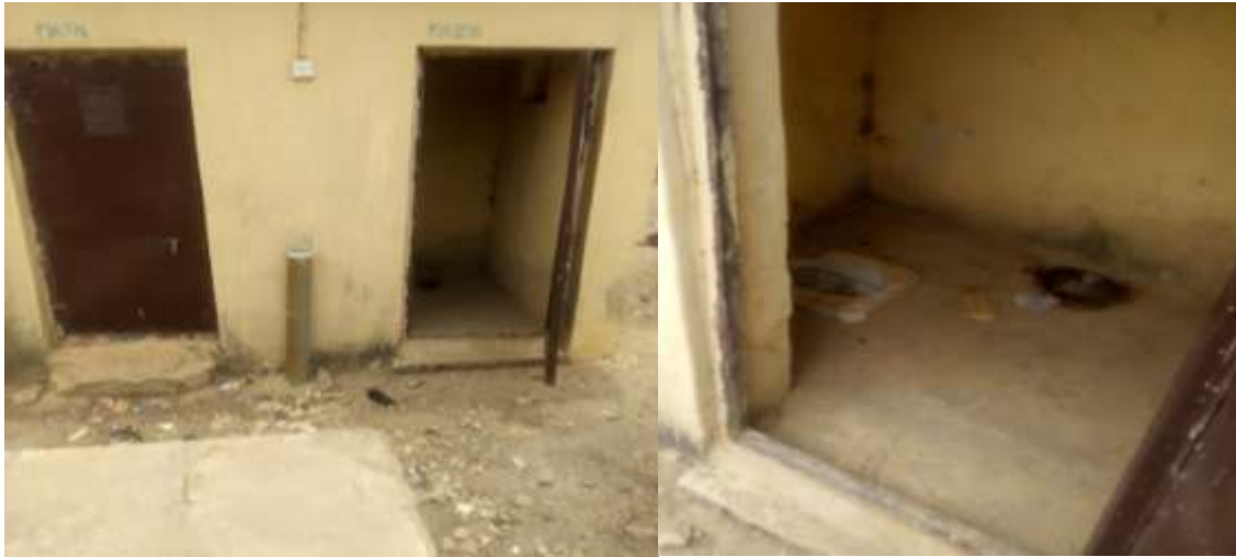
Picture 96: Dirty Toilets not in use due to Blocked Sewage System
