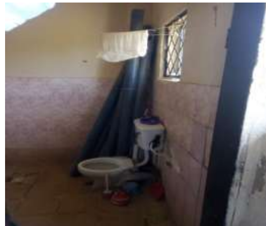
Picture 26: The only available Toilet
