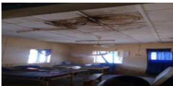
Picture 75: the Leaking Roof
